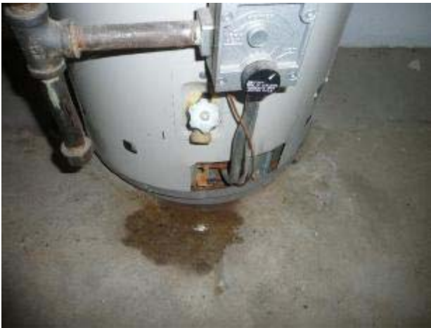
Leaking drain valve, missing flame guard
