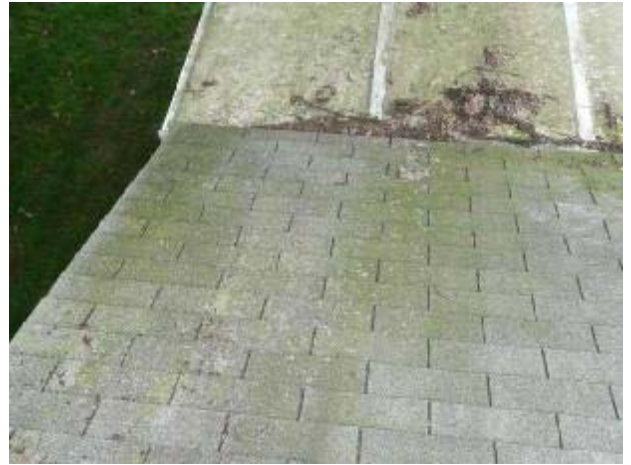
Algae and debris at the roof
