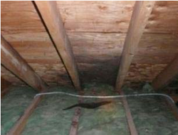
Mold above the bathroom
