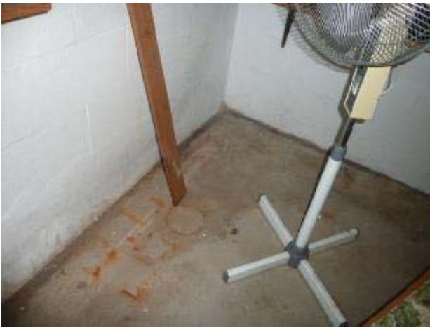
Evidence of moisture entry at the right side
