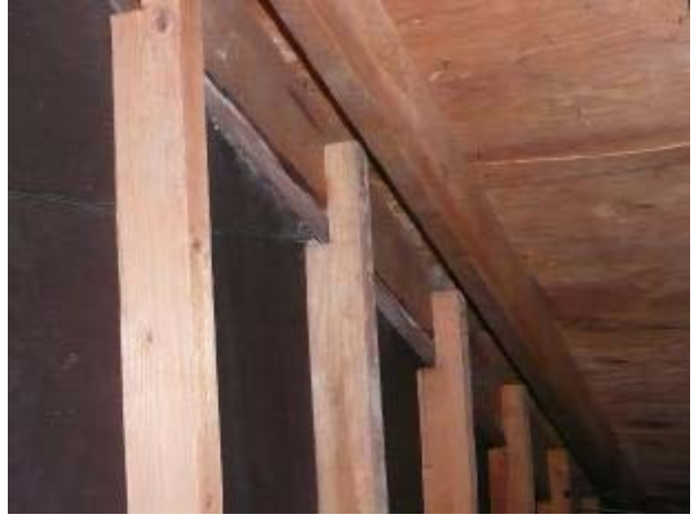
Smaller areas of staining at the chimney area.
