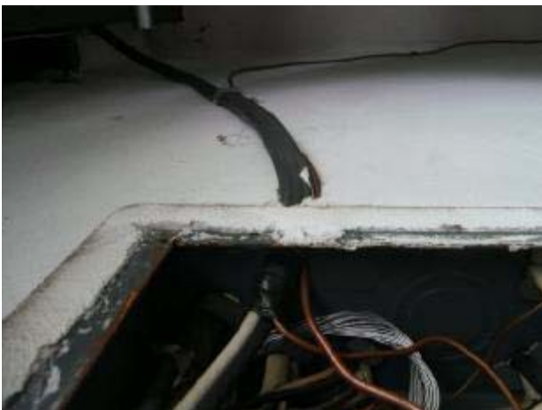
Improperly routed electrical wire.
