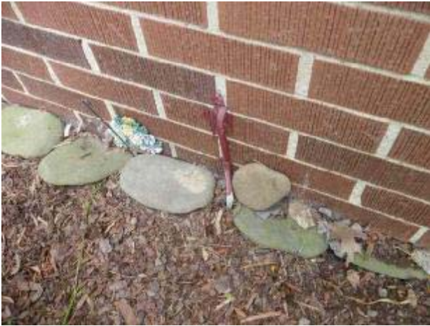
Exposed electrical wire at ground level
