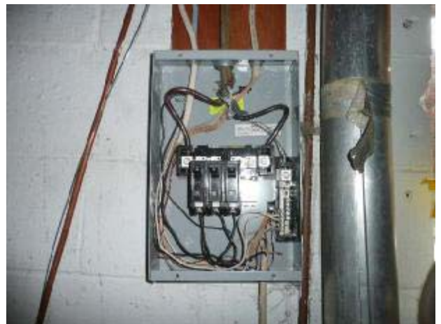
Basement sub panel.
