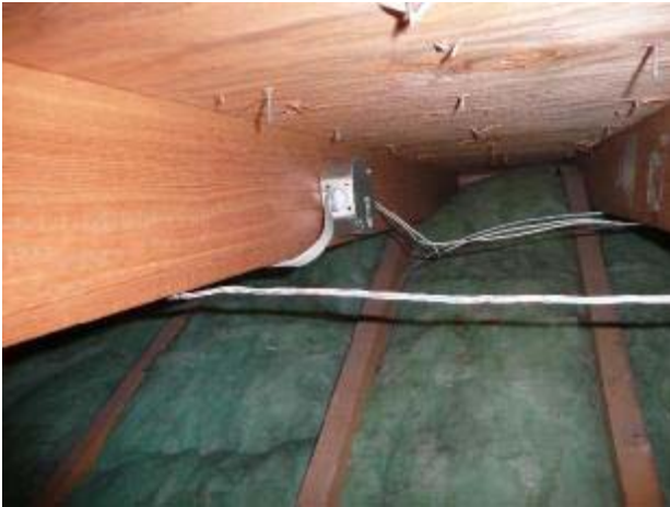
Improper wiring found at the garage attic.
