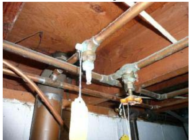
Example of corrosion at supply lines
