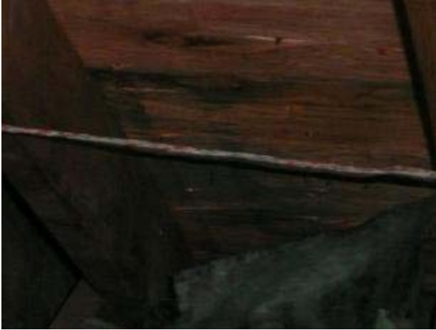
Smaller area of mold found at left rear corner of the garage attic
