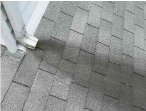
Downspouts discharge onto lower roof surfaces.
