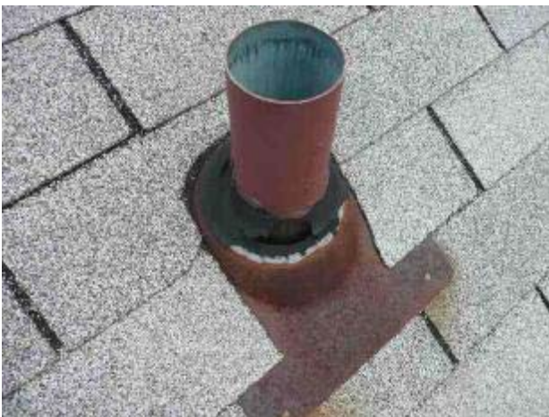
Separations at plumbing flashings and exposed nail heads.
