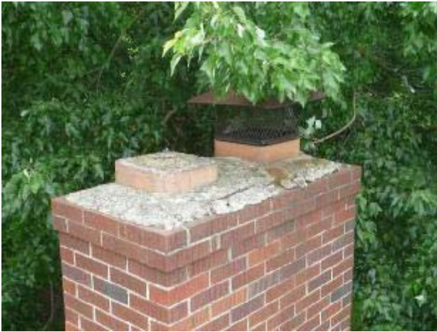
Deterioration at the mortar chimney cap
