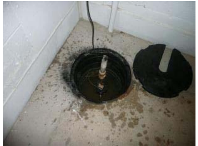
Water removal system
