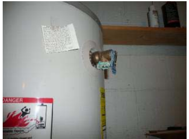
Evidence of leakage at TPR valve, missing TPR pipe
