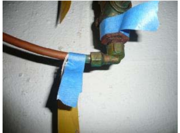
Compression fittings at the dryer branch
