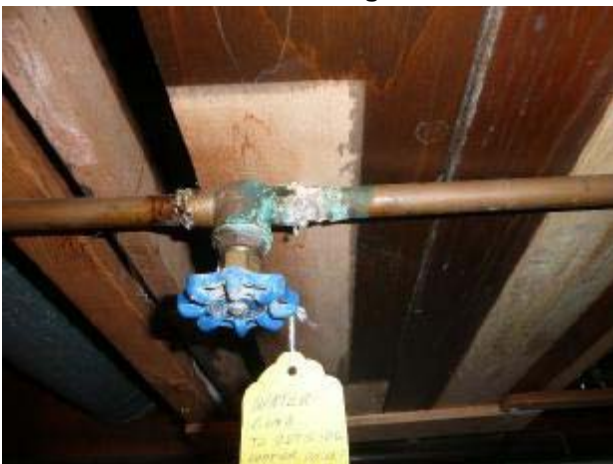
Example of corrosion at supply lines
