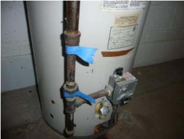
Example of gas leaks
